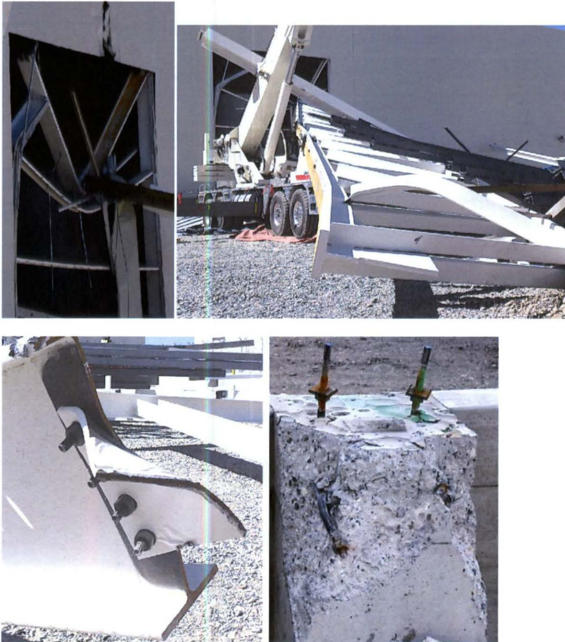
Figure 3: Examples of damage to OSE2 and adjacent building
