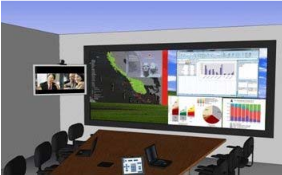
Conference systems allow for “Decision Rooms” where offshore and onshore staff, contractors and regulators can meet in a common place for superior team-based decisions
