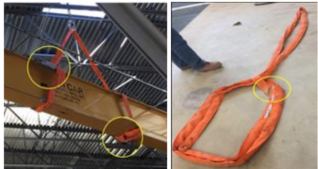
Photos showing sling failure that caused girder to drop
